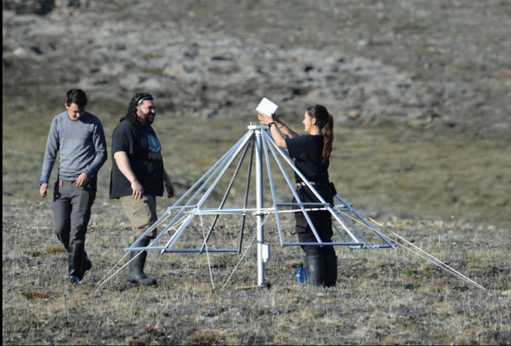
Long Wavelength Array (LWA) antennas;
